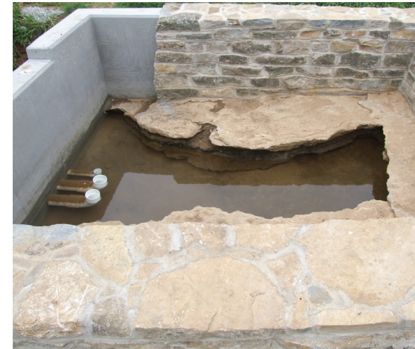
After the initial development, there is no cost to operate a gravity-fed spring
